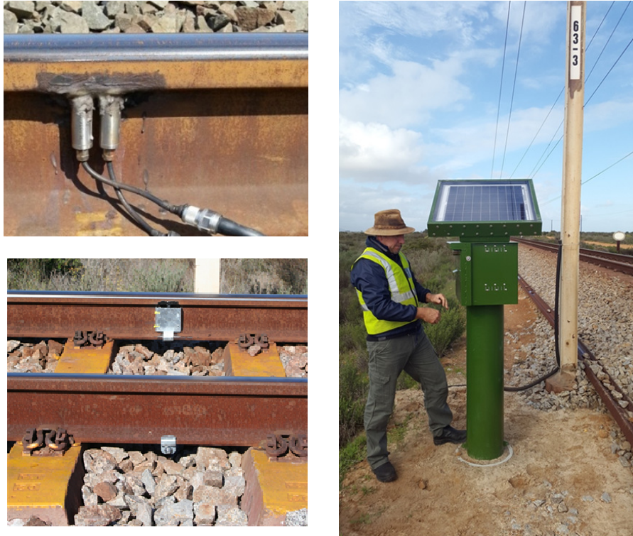
Fig. 5. UBRD Version 5 Transducers and Test Installation.
